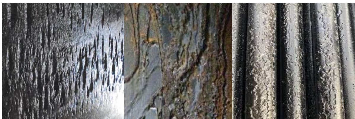
Photo. 4.7. Forms of damage to amine washing installations
