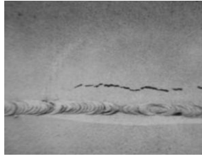
Carbonate cracking in a vicinity of weld
