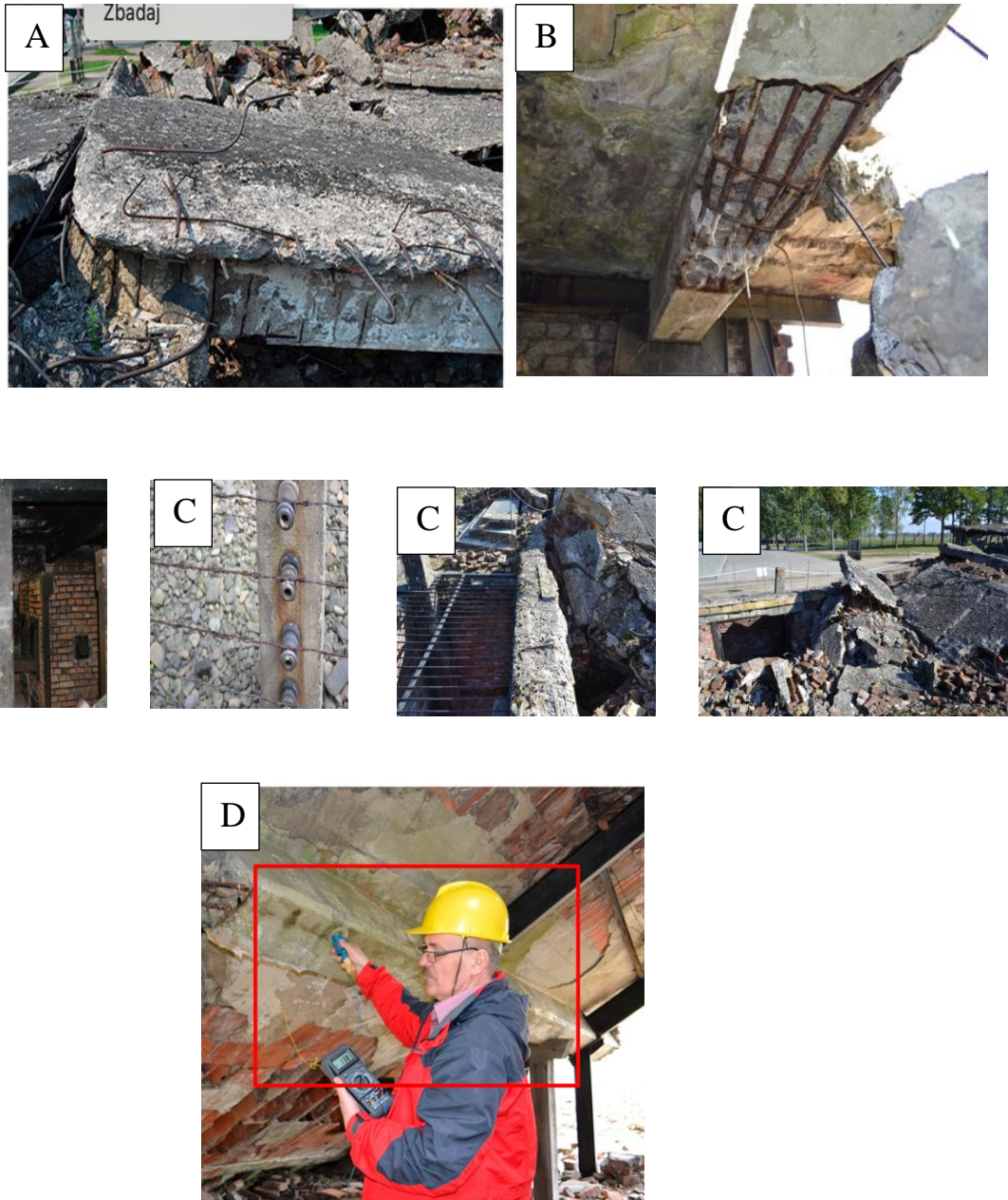
Photo. 4-5. (a) Exposed reinforcing bars of the ruins of crematorium no. 2 in Auschwitz II-Birkenau, (B) Ceiling of the gas chamber of this crematorium, (C) Typical forms of damage to concrete structures, (D) Recording a map of electrochemical potential on a reinforced concrete ceiling beam inside the ruins of crematorium no. 2 in Auschwitz II-Birkenau
