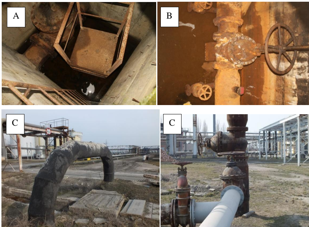
Photo. 4-13. (A) Condition of exemplary inspection chamber, (B) Corrosion condition of the fittings (gate valve), (C) View of the surface parts of the transport pipelines
