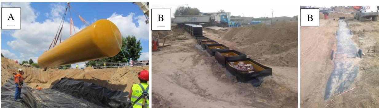
Photo. 4.19. (A) Fuel tank laid on plastic foil, (B) View of installed tanks of a fuel terminal
