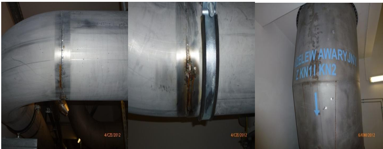
Photo. 4-16. Examples of corrosion damage to 316L steel localized in the vicinity of the welds in an ozonation station
