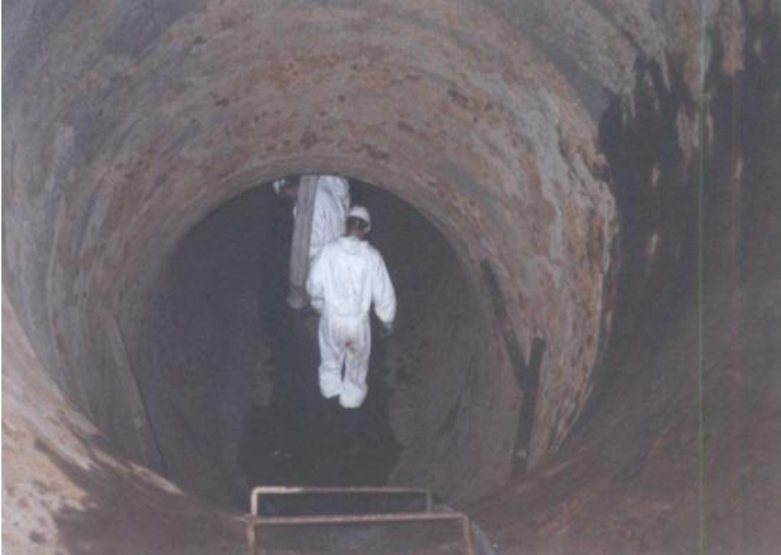
Fig. 4-17. Bełchatów Power Plant discharge pipeline and employees of the Department during corrosion inspection
