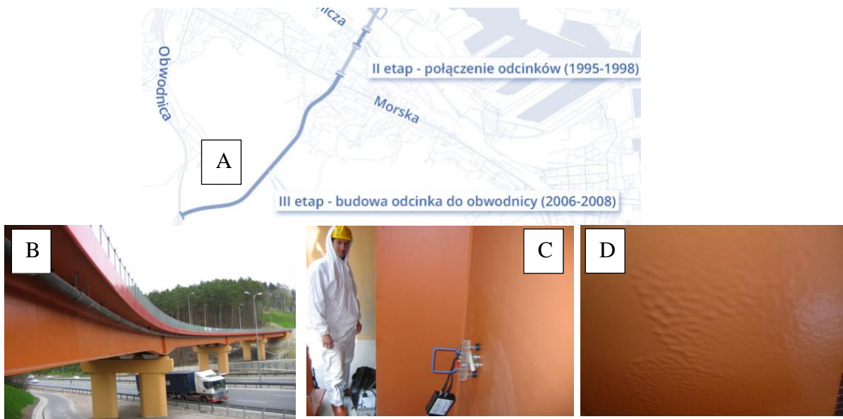
Photo. 2.2. (A) The course of the Kwiatkowski Route, (B) The view of the overpass over the ring highway, (C) Impedance measurements of the condition of the coating system, (D) Defects of the anticorrosion coating
