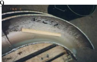
Erosion-corrosion damage to the elbow of the 5Cr alloy. Heater outlet
