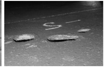
Craters at the bottom of the raw crude oil tank
